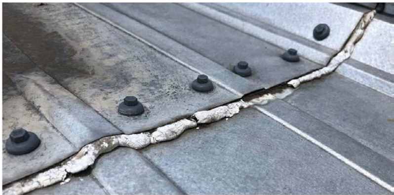
An example of a failing lap within a T-panel roof system with exposed fastener lap.
