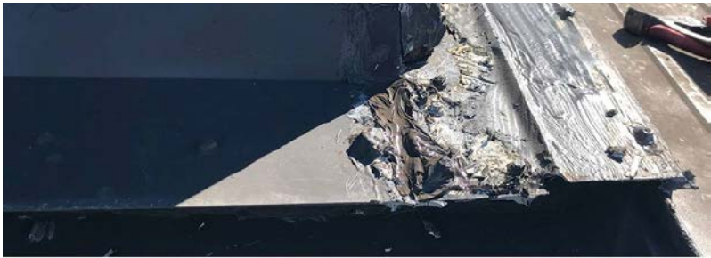
This industrial metal roof system failed multiple repair attempts. There was no deck or water-resistant barrier beneath the panels.
