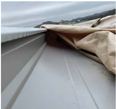
Example of damaged ribs on a metal panel; the waves in the ribs prevented a proper double lock.
